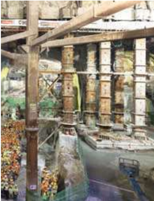
The cavernous Admiralty station box hosts a gathering of the staff involved in its excavation and construction
